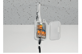
Pendant light connection in a suspended ceiling
