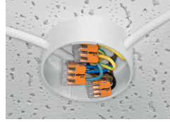
Lighting distribution in a ceiling canopy
