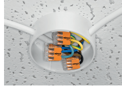
Lighting distribution in a ceiling canopy
